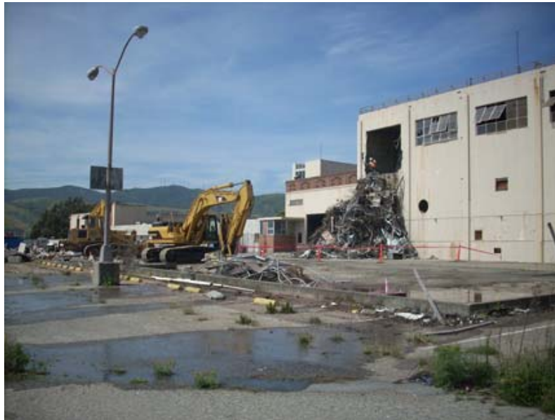
Pulvirizer tears down a building at the former Schlage Lock factory on Bayshore Boulevard.
